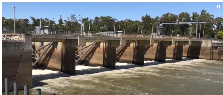
▲ Radial gates at Torrumbarry Weir on the Murray allowing a small and controlled downstream flow.
