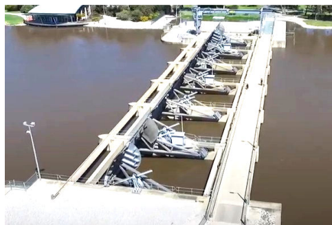
▲ Radial gates raised to full height allow open flow on the Murray River.
